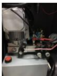
Picture 27 (oil tank)
