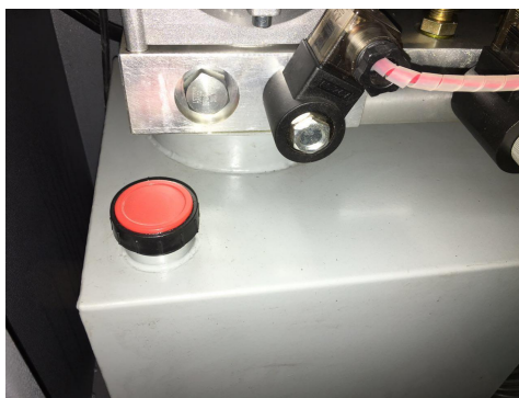
Picture8 overflow valve
