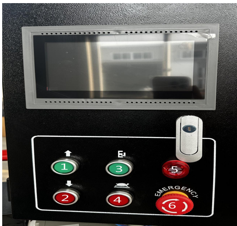
The physical control panel on each column.
